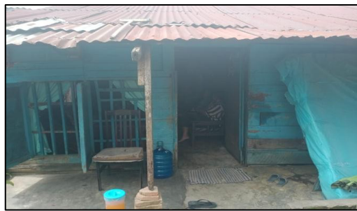
Figure 1. Condition of Payan Hutahayan House before repairs
